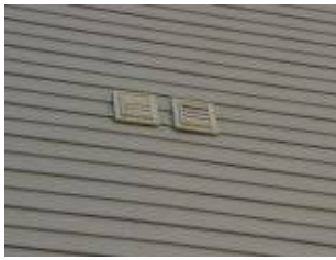
Photo 8 Reccomend additional Screening, prevent bird intrusion.
